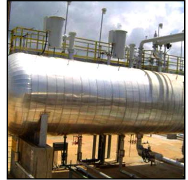
Exterior view of the coalescer.
