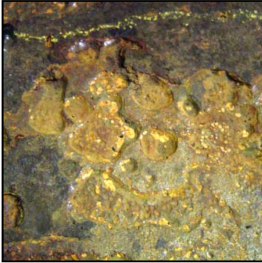
Extent of the corrosion due to the effects of the microbiological attack.
