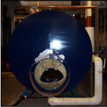
The tank inside the Powerhouse
