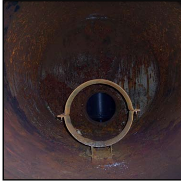
View of the internal corrosion
