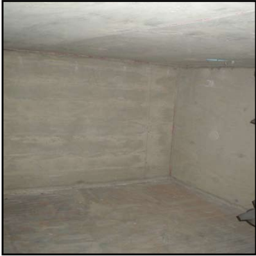
Bare unprotected mixing tank
